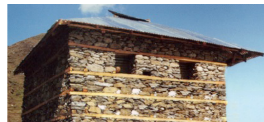
Figure 6. Bahitter Tarz-e-Tameer: horizontal wooden elements subdivide the height of the wall and break its monolithic character when it collapses during an earthquake.
