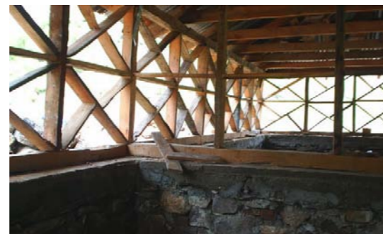
Figure 5. Construction process of the Kot Dhiji method using wooden diagonal bracings in walls for reinforcement and earthquake resistance.
