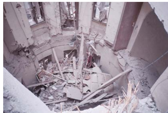
Figure 2. Damage to buildings caused by severe bombing, Belgrade.
