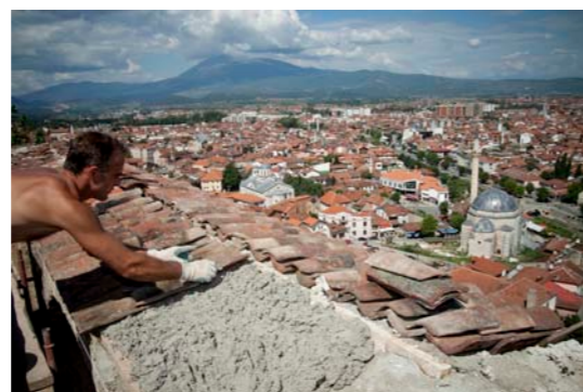
Figure 4. Restoration works on the 19th-century structure. Copyright of PSF. Credit: Arno Fougères 2010.
