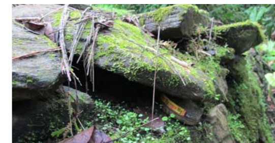
Figure 5. Detail of the damage caused, park of Ciudad Perdida.
