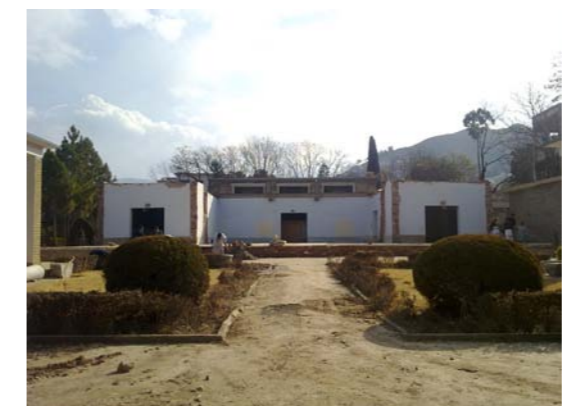
Figure 6. Ongoing reconstruction and rehabilitation of Swat Museum by the Italian mission following the damage.
